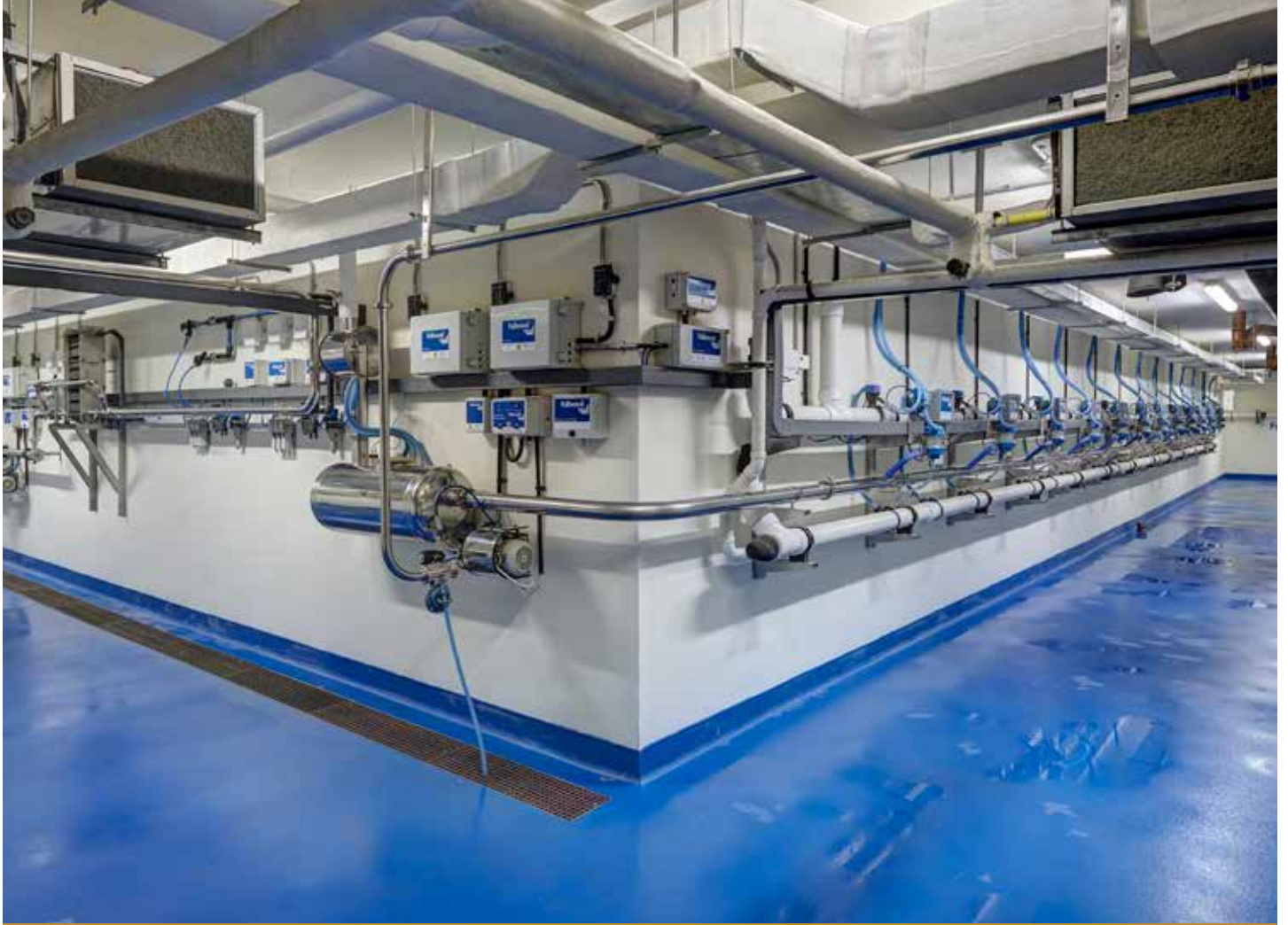
CELLAR MILKING SYSTEM
